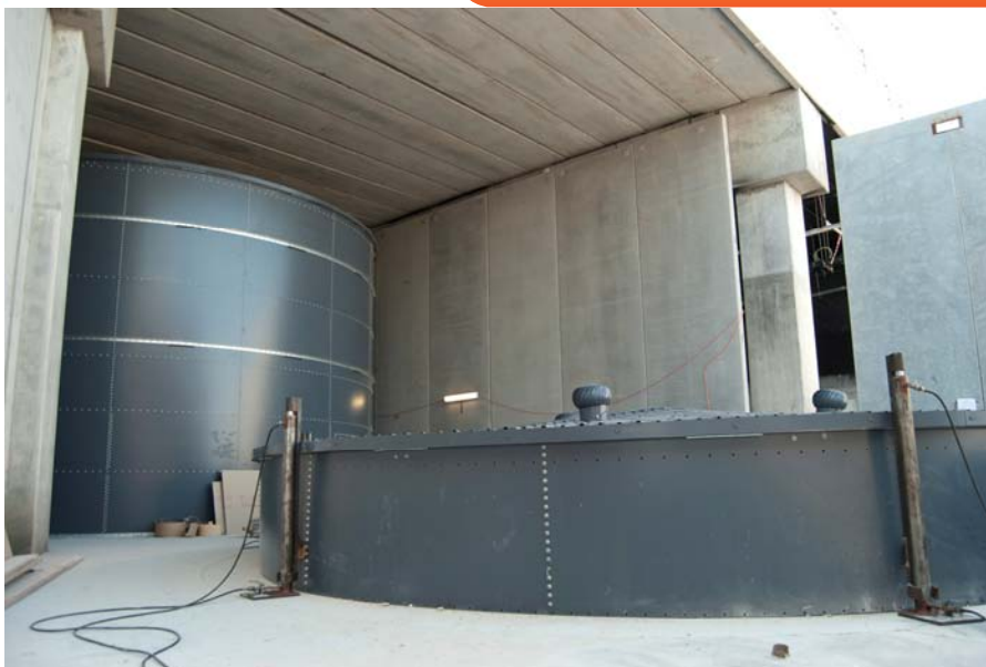
Fire deluge tanks
