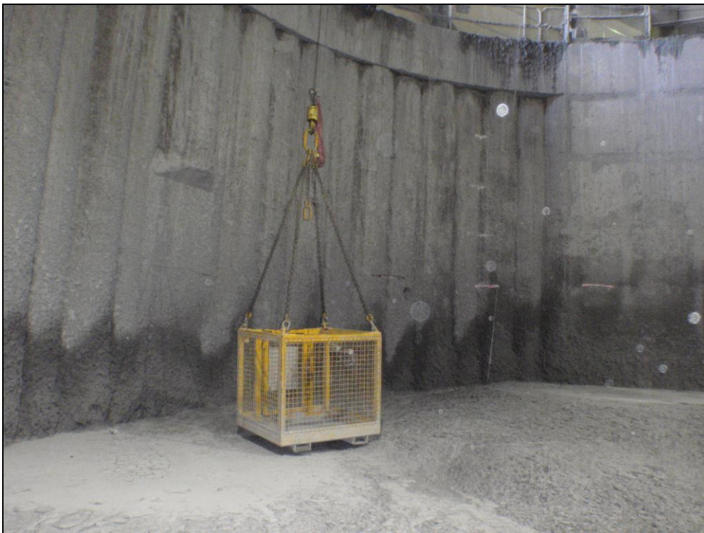
Shaft backfill progress: Shaft prior to dirt and rock backfill and breaking back of piles
